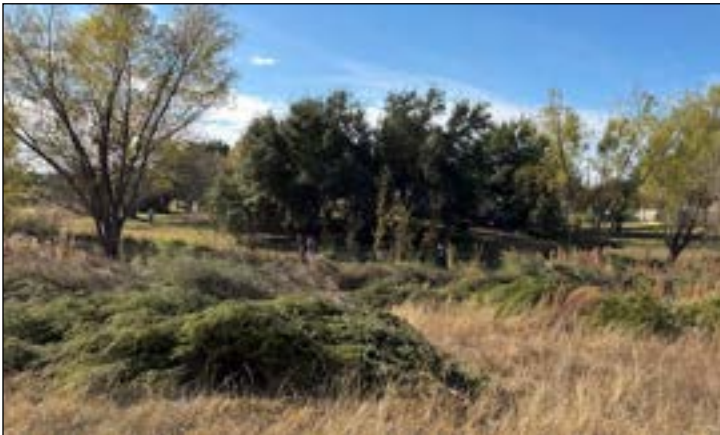
The work area after clearing. Note the piles of cut material that will be chipped and used as mulch.
